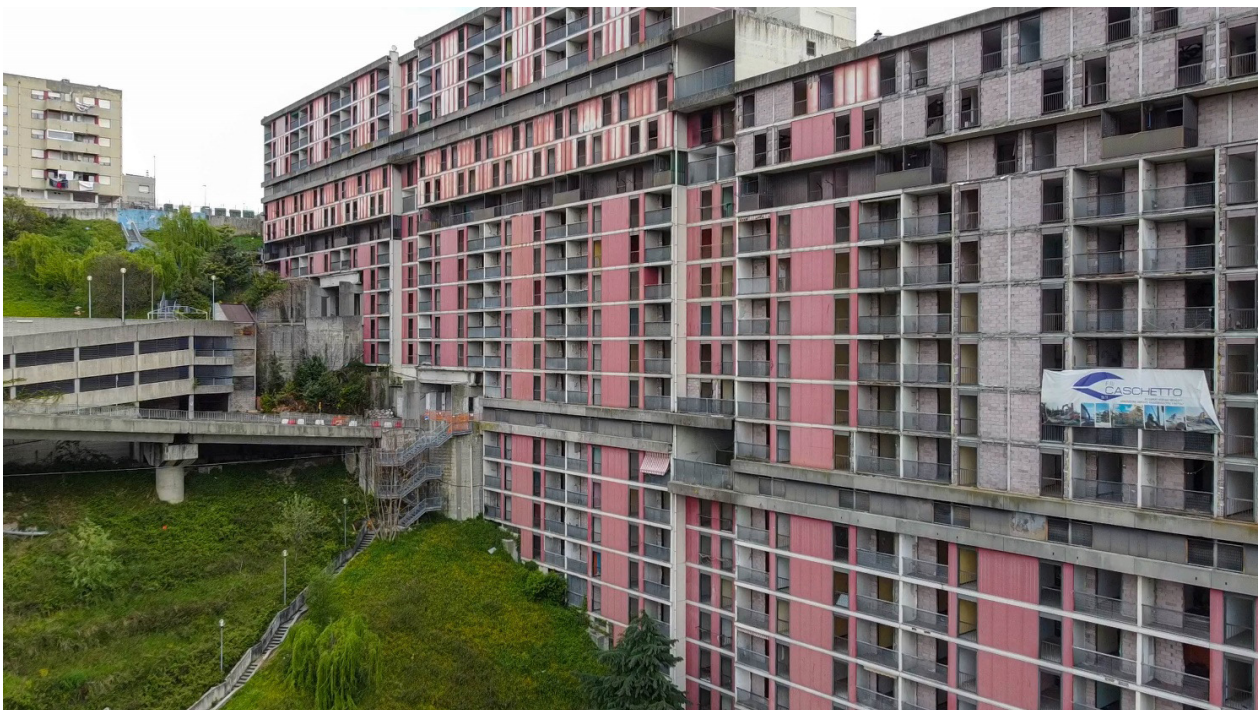
Figure 5. The facades of the red and white Begato Dam during dismantling and demolition, 2021.
