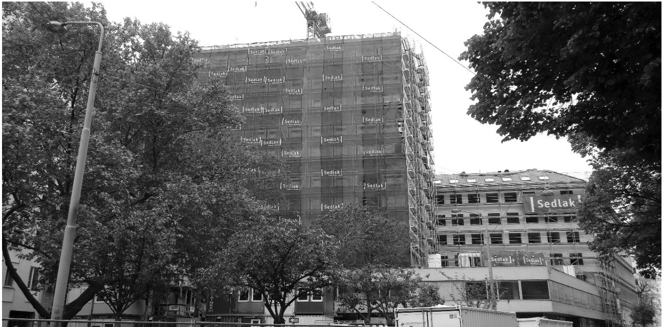
Figure 4. Traditional centrally located NP student accommodation from the 1970s under renovation. Source: Photograph taken by Elisabeth Gruber, 2021.
