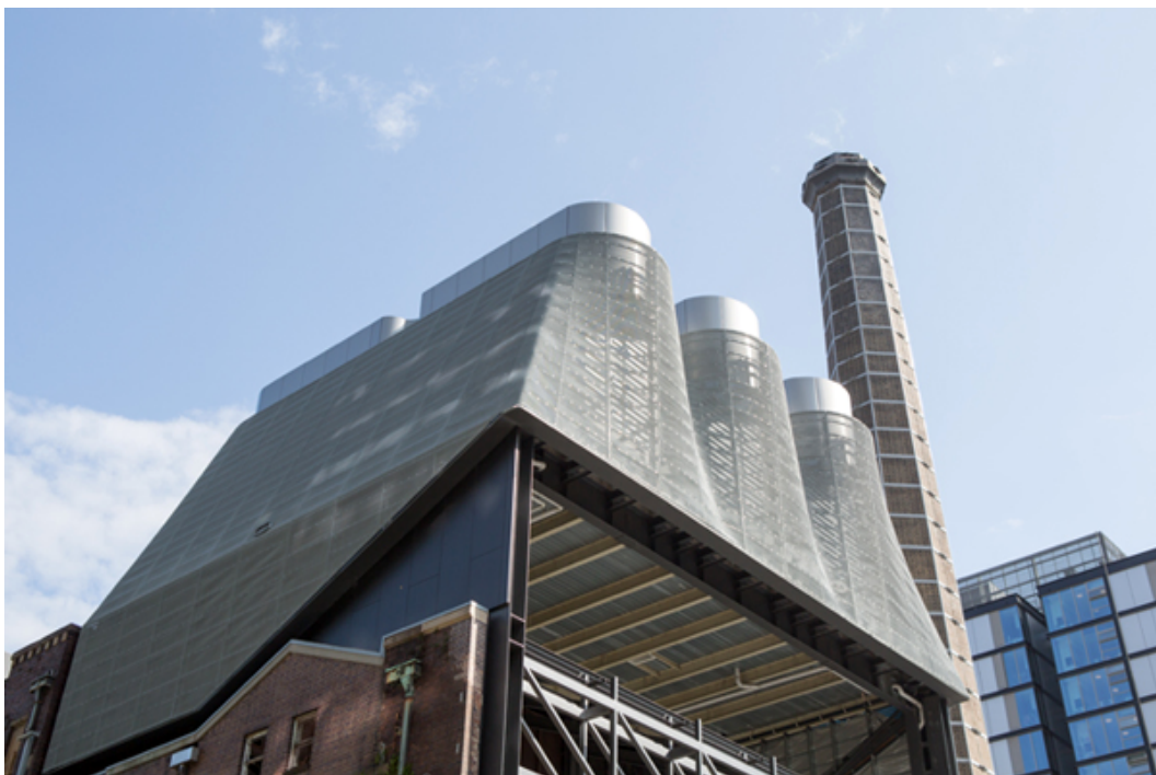
Figure 4. Cooling towers of the Trigen-plant. Credit to Shane Lo.
