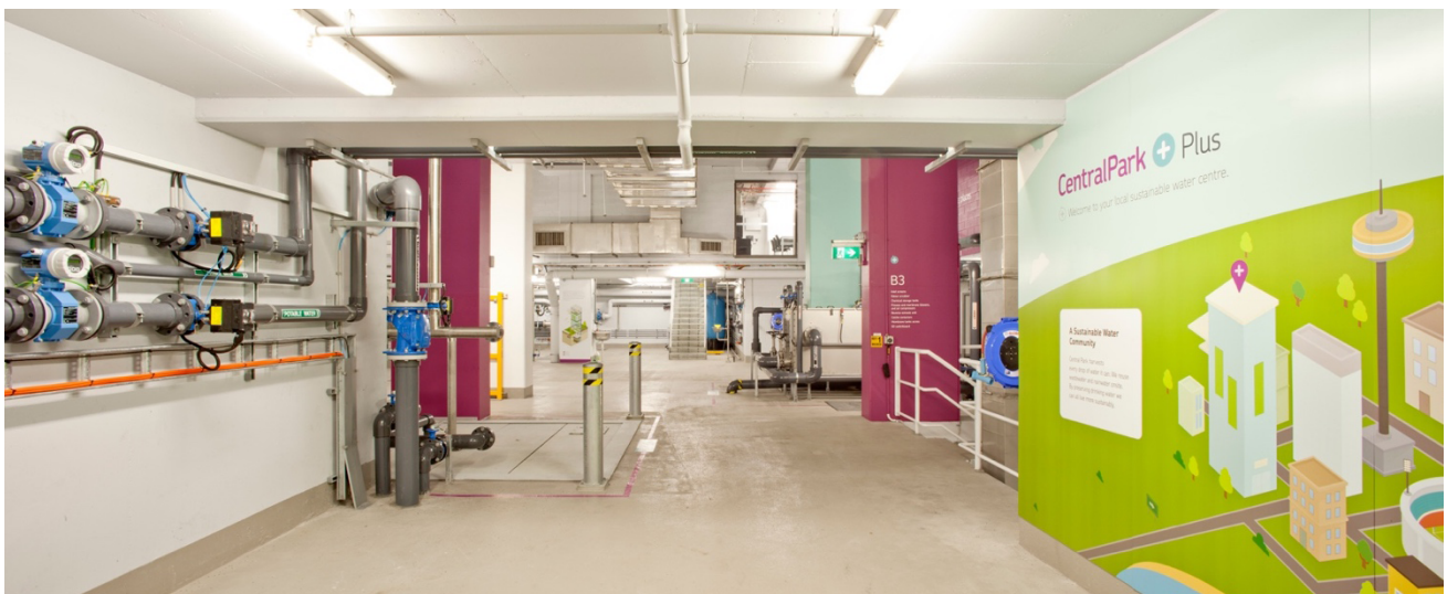
Figure 2. Central Park Plus: The world’s biggest recycled water centre at the basement of a residential building. Source: www.centralparkplus.com.au
