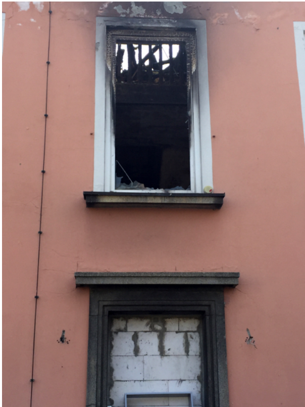
Figure 11. The burned out Husarenhof Hotel in Bautzen, originally intended for refugees. Photo taken by Hajo Neis, August 2018.
