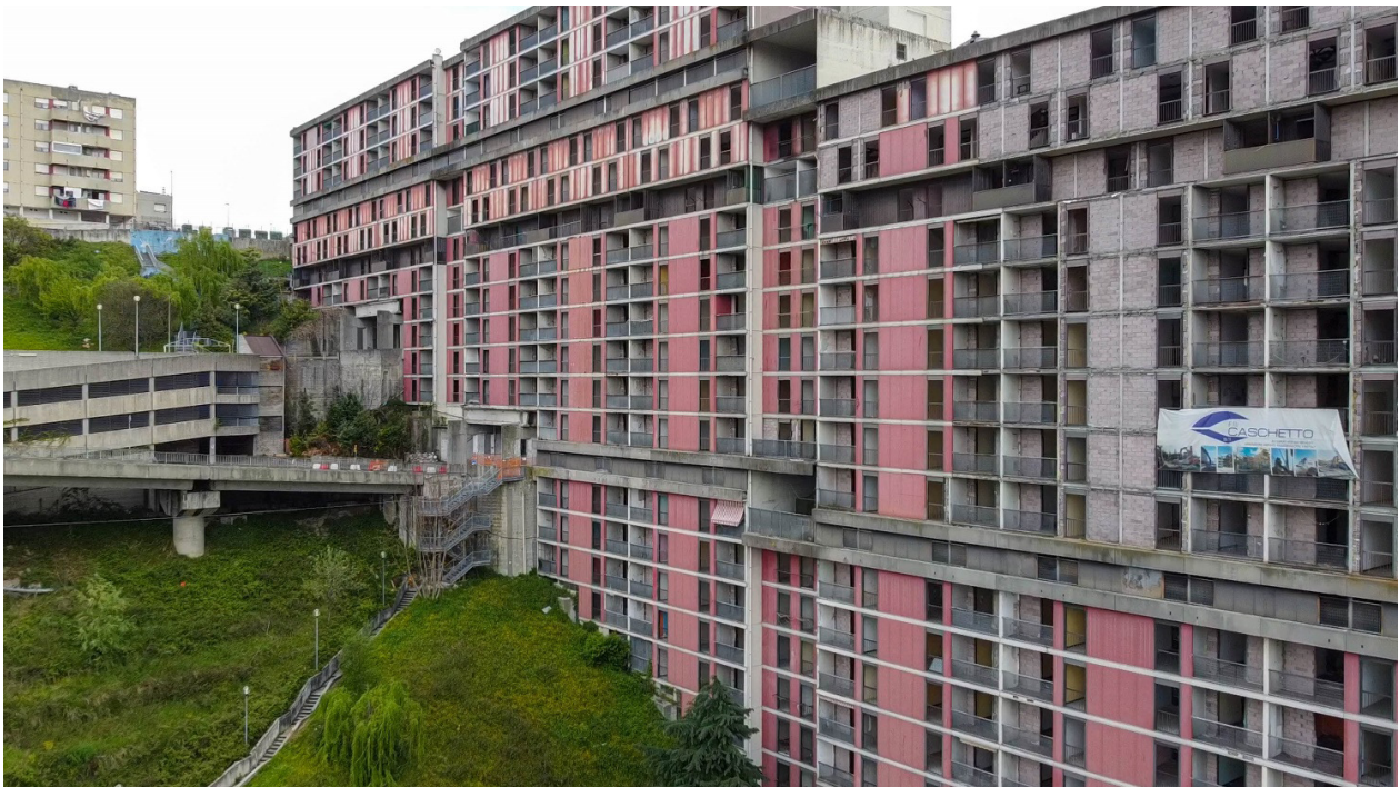
Figure 5. The facades of the red and white Begato Dam during dismantling and demolition, 2021.
