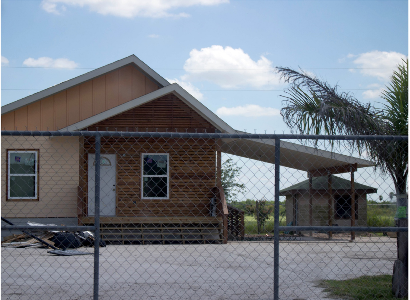
Figure 3. Nearly completed RAPIDO prototype home, designed using a sustainABLEhouse model, under construction in a colonia north of Weslaco, Texas. Source: Author (2015).
