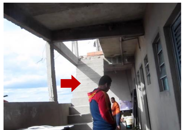
Figure 17. Case B, unfinished building. The arrow calls the attention to the stairs to the third floor, with no protection. Source: author's archive, 2013.
