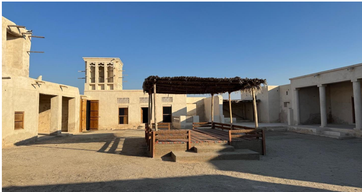
Image 18: the ongoing renovation works at Al Jazeera Al Hamra of Ras Al Khaimah
